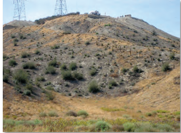
Figure 1 — Pre-construction location of the El Casco Substation within the Norton Younglove Preserve. Geologists identified a layer of clay within the hillside. Removal of the toe of the slope increased the likelihood of slippage. Therefore, a tension cable anchor system was installed during construction.
