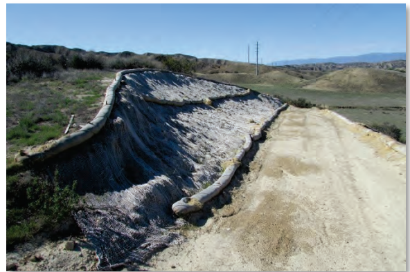
Figure 31 — View of subtransmission restoration site 36. Note the lack of plant cover and container plants. March 12, 2014.
