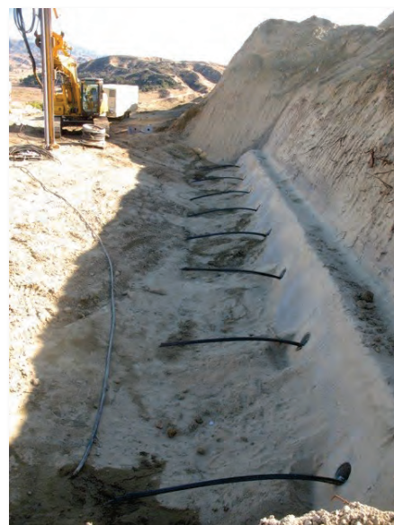
Figure 4 — A tie-back wailer under construction on the face of one of the terraces. After completion of the wailer, the 120-foot cable anchors were placed under tension.
