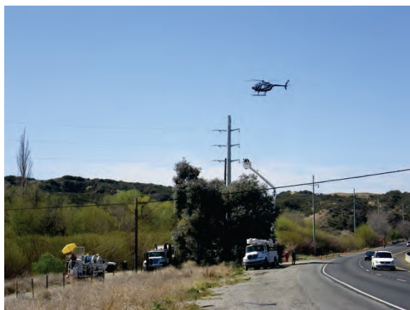
Figure 20 — View of crews installing conductor along Segment 7 adjacent to Highway 60. The photograph faces west.
