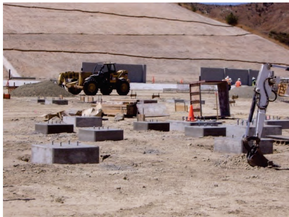
Figure 8 — At the El Casco Substation site, crews worked on foundations for the AA banks for the 220 kV switchcracks. The photograph faces south.
