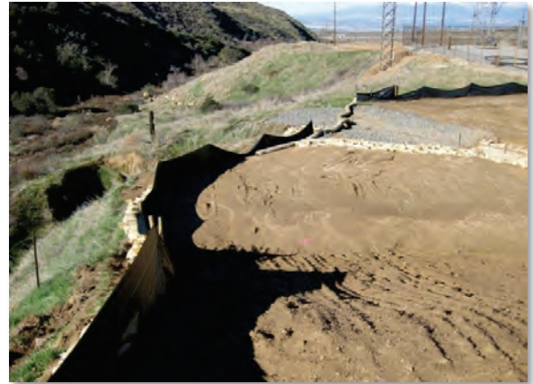
Figure 24 — Erosion control devices mostly prevented siltation into a nearby watercourse during storms at Zanja Substation. The photograph faces west.
