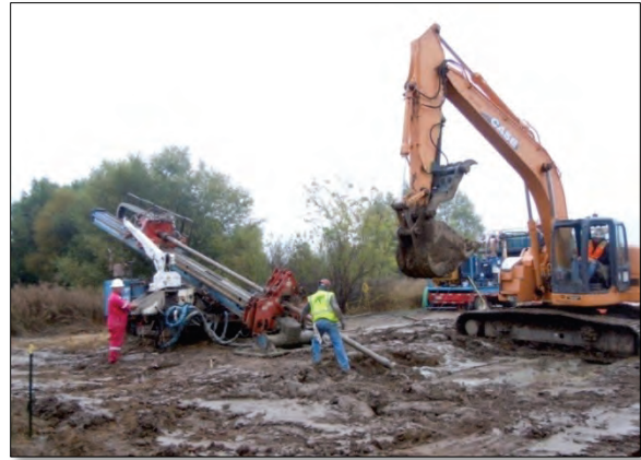
Figure 10 — Along San Timoteo Canyon Road, the drilling rig at the bore entry side.
