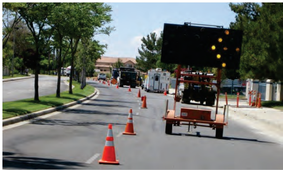
Figure 27 — Proper signage, demarcation of the work limits, and traffic control at the Sun Lakes Blvd FOC installation. Steel plates protect the road surface and cover open trench.
