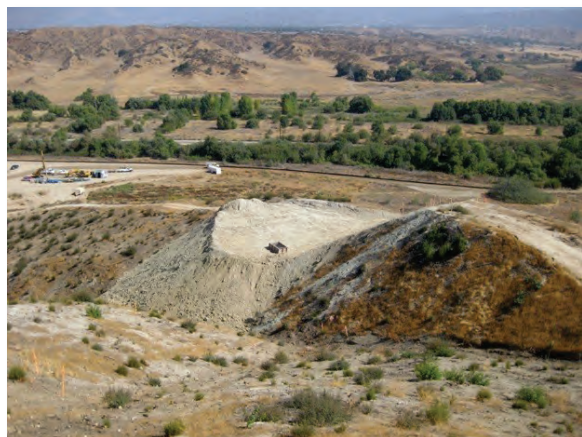
Figure 3 — Beginning terracing work in stair step fashion. There were eventually four terraces on the ridge in view. The photograph faces north.
