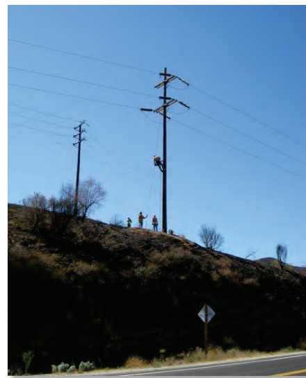
Figure 26 — FOC installation work between Mentone and Zanja Substations. Linemen climbed the poles in areas too remote for a bucket truck to approach.
