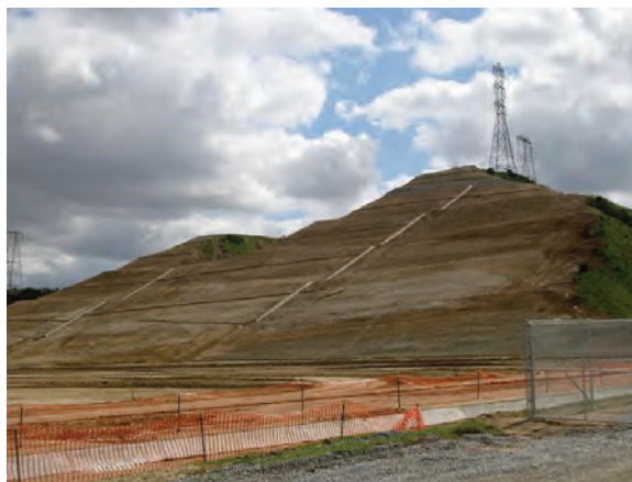
Figure 6 — View of the completed terraced slope at El Casco Substation. Note the newly installed V-ditches. The photograph faces southeast.
