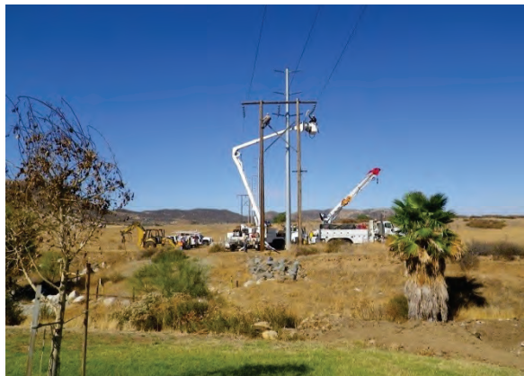
Figure 21 — View of crews removing an old wooden pole from Segment 2 and rerouting the old conductor to the new steel pole. The photograph faces west.
