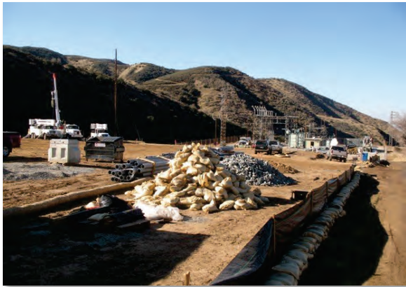
Figure 23 — Expansion and upgrading of the Zanja Substation. The slope east of the substation was removed and spread on adjacent SCE land. The photograph faces west.
