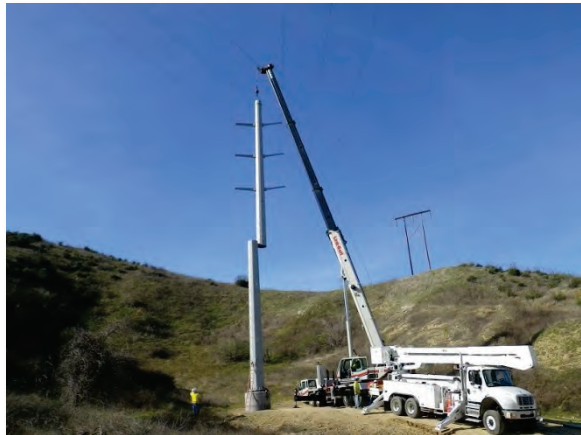
Figure 19 — View of tubular steel poles being installed just south of the El Casco Substation. The photograph faces southwest.
