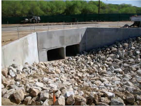
Figure 7 — View of completed box culvert inlet near El Casco Substation entrance. The photograph faces north.
