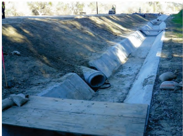
Figure 11 — View of installed wildlife culverts under the main El Casco Substation access road. The photograph faces east.
