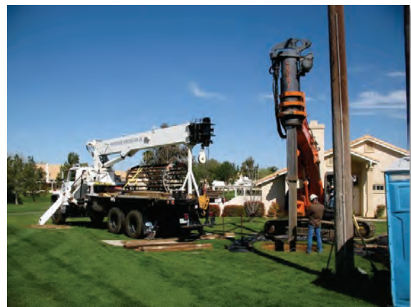
Figure 18 — View of crews installing new pole foundations for Segment 3 of the subtransmission line through the Sun Lakes development. The photograph faces northwest.
