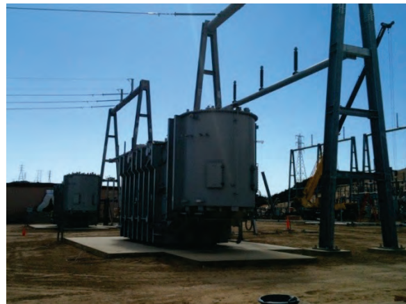
Figure 9 — At the El Casco Substation site, a second 220 kV transformer was delivered on August 17.
