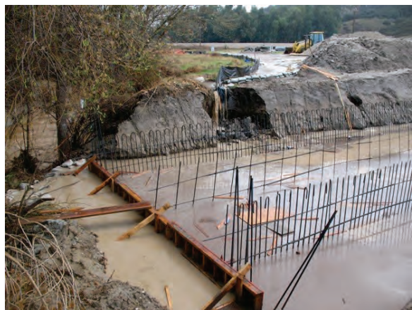
Figure 5 — The partially completed box culvert at the El Casco Substation access road was inundated with stormwater, which then poured into San Timoteo Creek. The photograph faces southeast.
