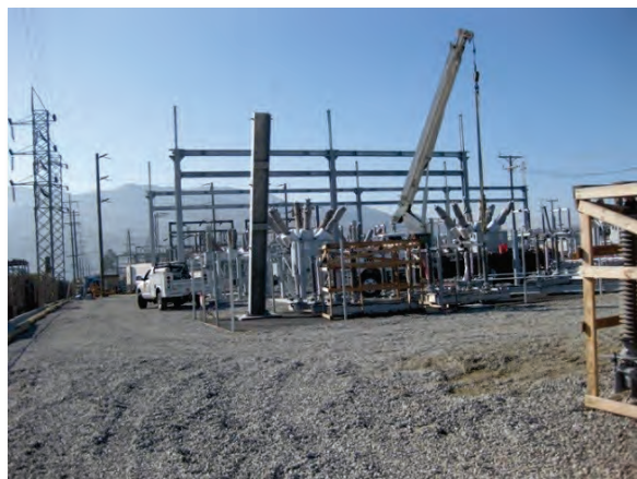
Figure 25 — Circuit breakers and other electrical equipment were installed in the northern portion of the Banning Substation site. The photograph faces south.
