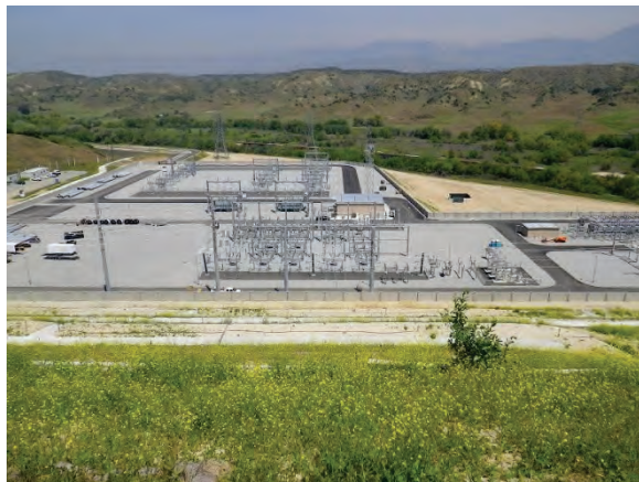
Figure 17 — View of El Casco Substation. The photograph faces north.
